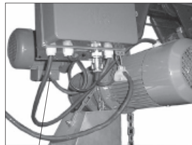
Connection of cable from controlbox in to junction box on motor.
